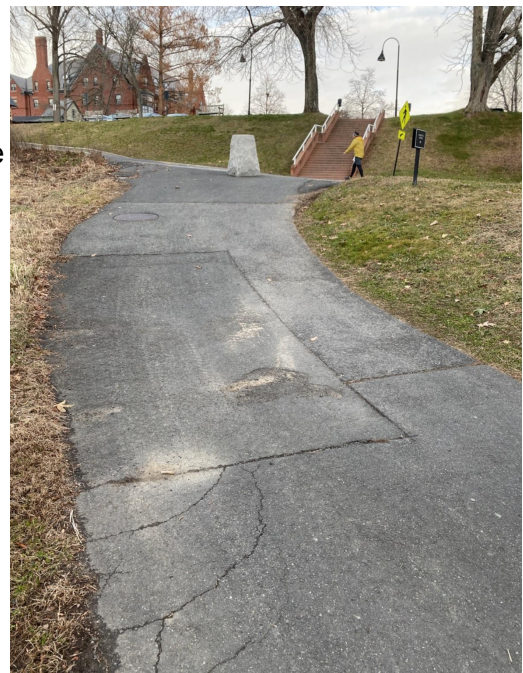
Figure 9 (right): An image of the path leading down to the athletics field. This path is a problem because it both has a slope of 9.8 degrees, way above an accessible measurement, and it lacks a railing.
